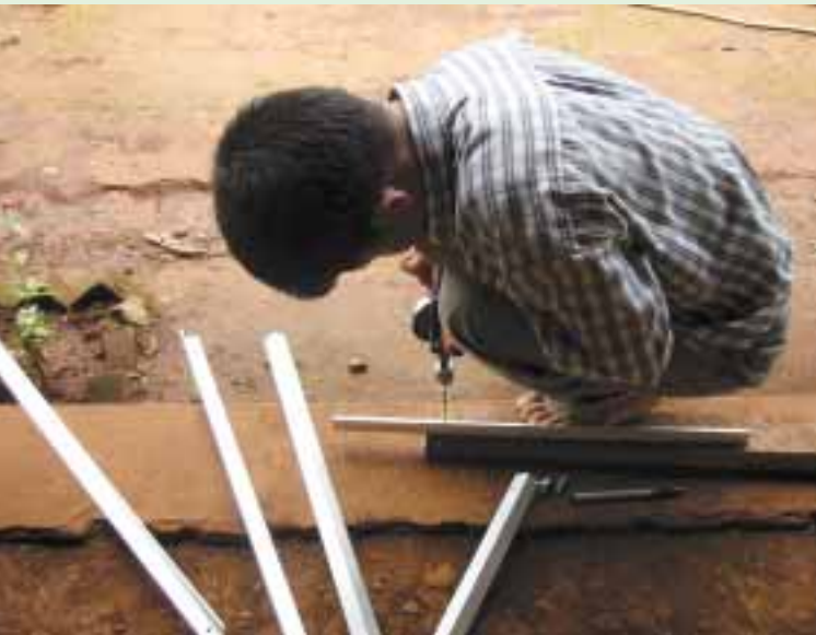
Low tech supports high tech—building a PV mounting rack with hand tools.
