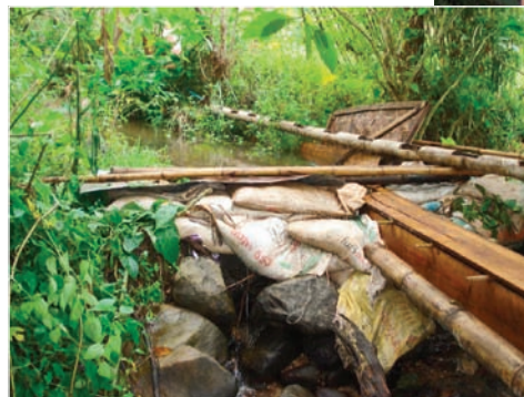
Below: Local lumber, rocks, sandbags, and bamboo were used to construct the weir and waterway.
