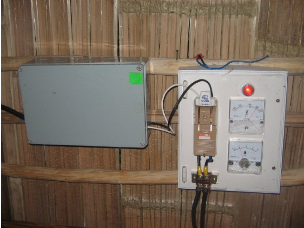
Figure 15: capacitor box and switch box at the power house. When the photo was taken the generator was generating 4 amps at 400 volts. We were able to push it to 7.5 amps (3 kW) but have decided at this point to let more water flow in the stream since the village does not yet need more than 1.6 kW.
