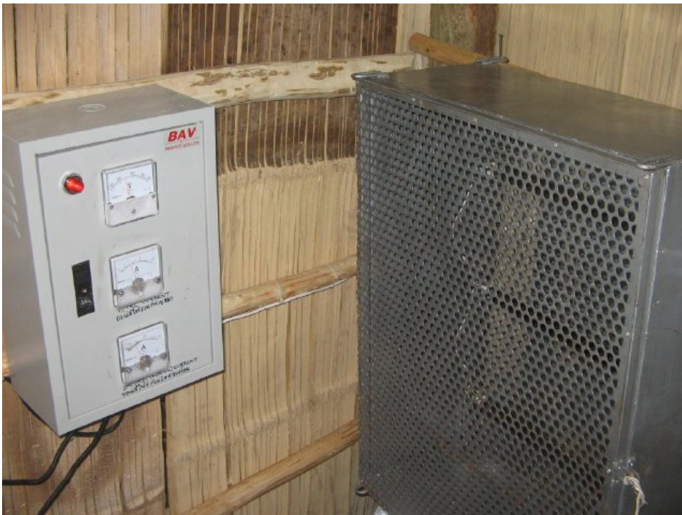
Figure 16: ELC and ballast load in metal cage.
