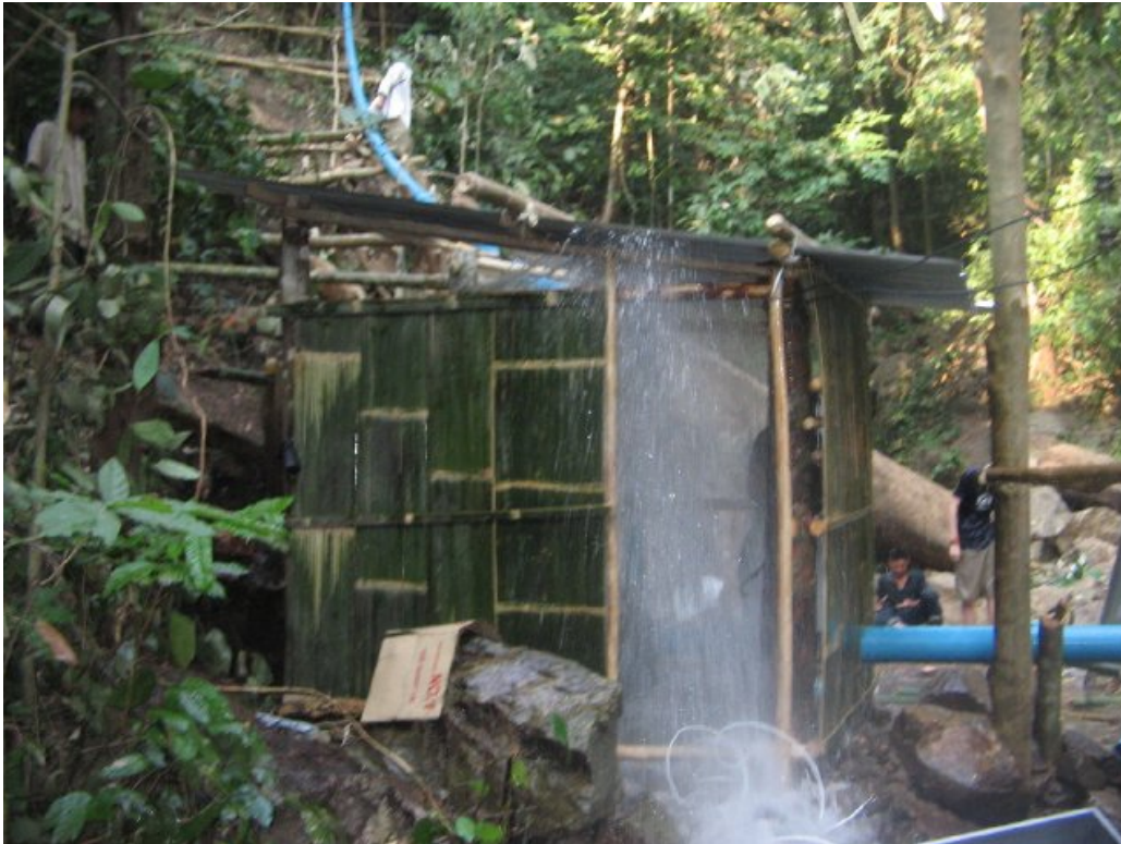
Figure 13: Poor communication and a bad glue joint led to a nearly disastrous pipe rupture inside the powerhouse, completely drenching all the electronics and tools. Amazingly, no one was hurt and almost of all of the electronics were unharmed.
