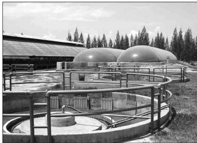
This biogas digester produces 500KW for a Thai farm.
