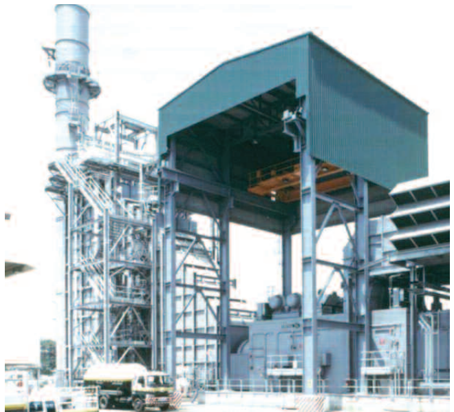
A 113 MW CHP plant sells power to EGAT, the state-owned utility (Bangkok Cogeneration)
