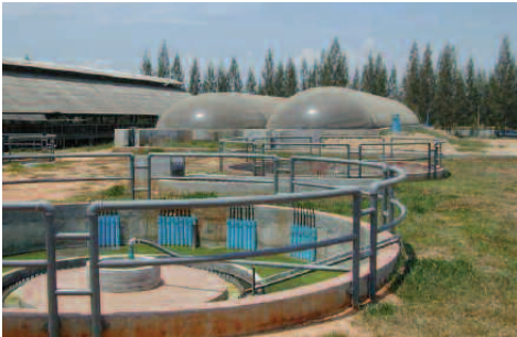
Biogas digester at SPM farms produces enough gas for 500 kW of generation (EPPO)
